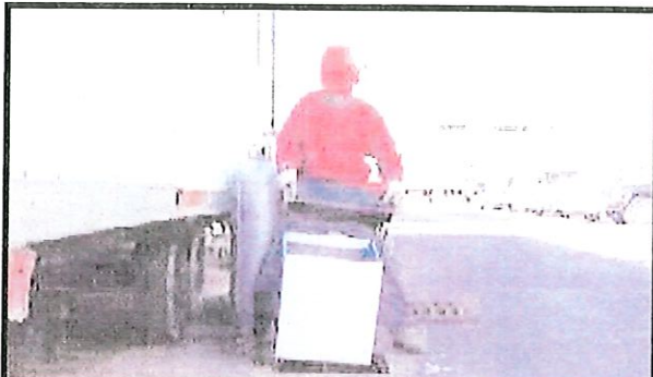
A worker inserts a catch basin insert for oil and grease, trash, debris, and sediment removal from storm water as it enters the storm drainage system (Source: AbTech Industries, 2001)
