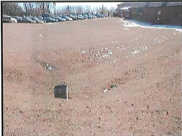
Infiltration basins are designed to collect storm water from impervious areas and provide pollutant removal benefits through detention and filtration
